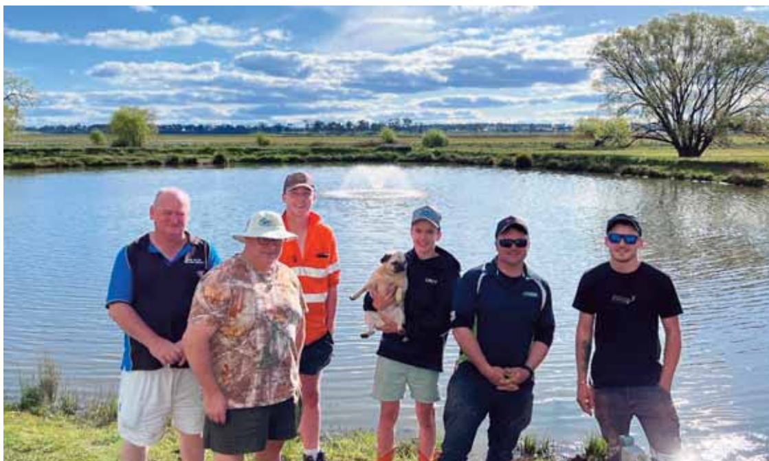
AERATOR INSTALLED: David Wilcox, Grant Roberts, Ryan Jones, Brock, Adam, and Brodie Hoffman
