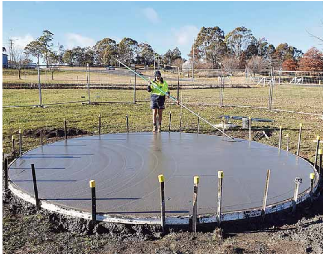
The slab has been laid this week for the planned Mandala Garden
