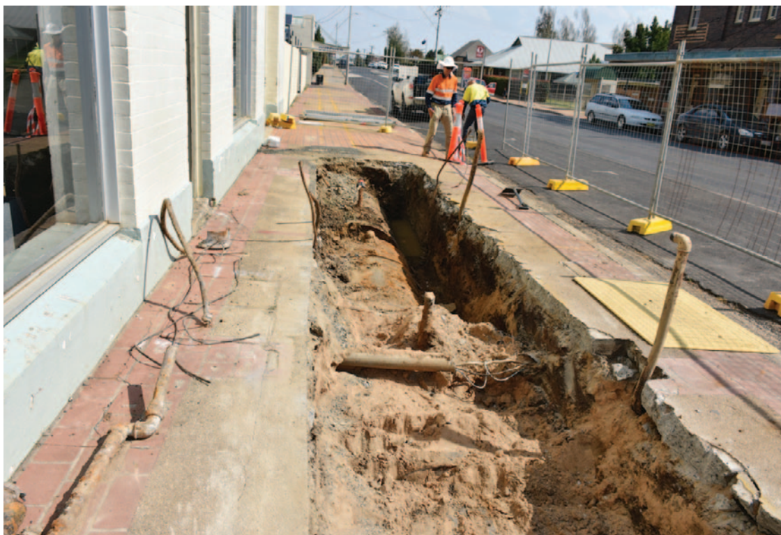
The previous stage of the project encountered significant delays and additional costs after underground fuel tanks were discovered beneath sections of the footpath.
